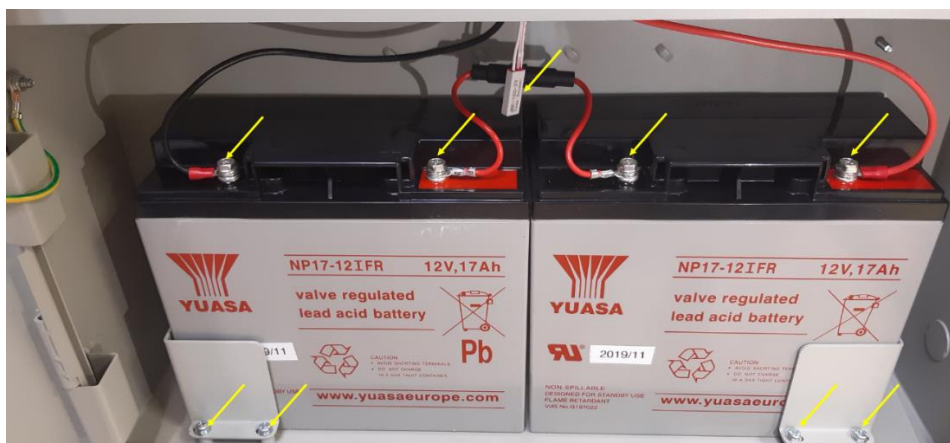
Figure 9: Battery Connection Location for 17 Ah
