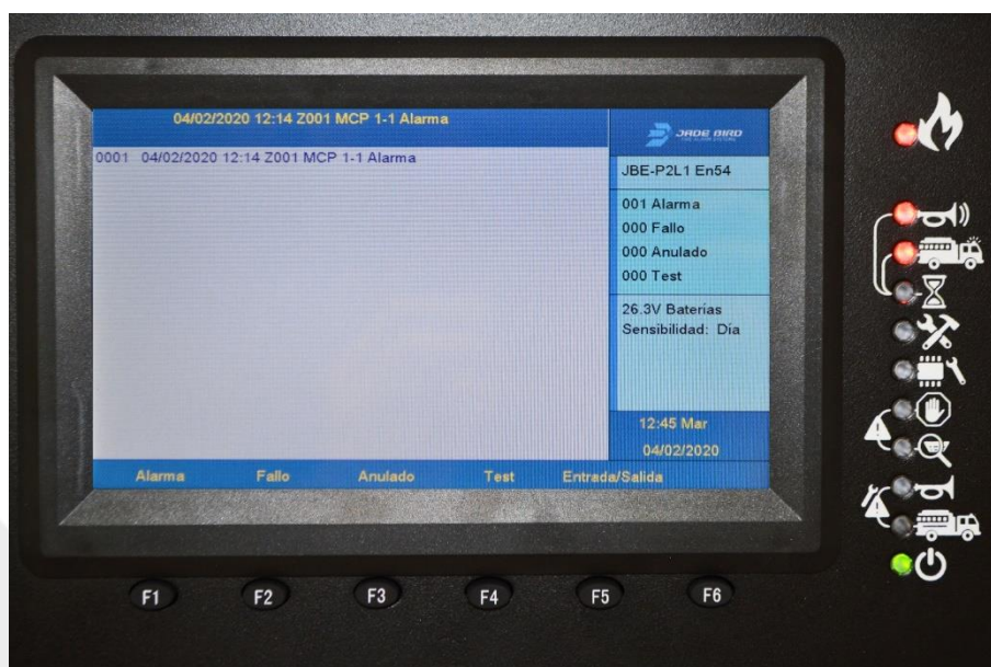
Figure 20: The alarm screen
